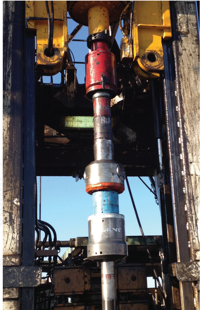
weCATT™ in operation with CRT
